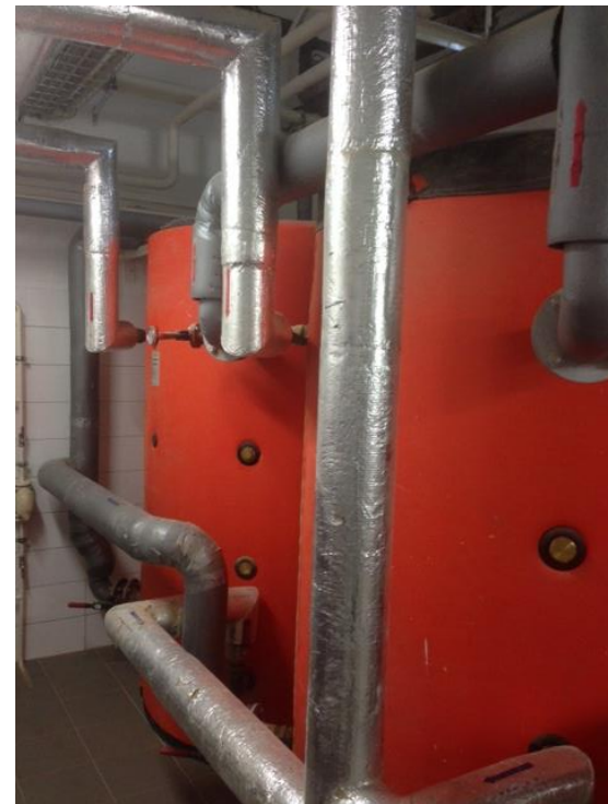
Hot water storage tanks
